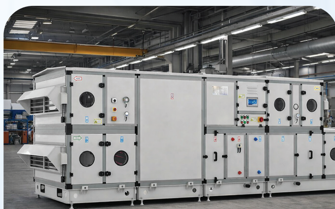
Air Handling Unit
