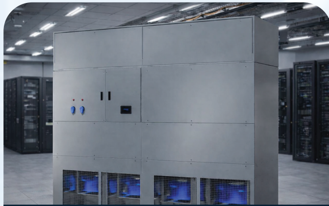
Computer Room Air Conditioning – CRAC / CRAH
